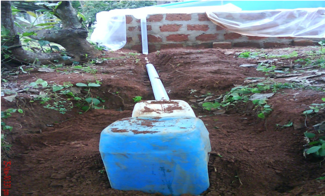
Plate 4.4 Underground recharge system
