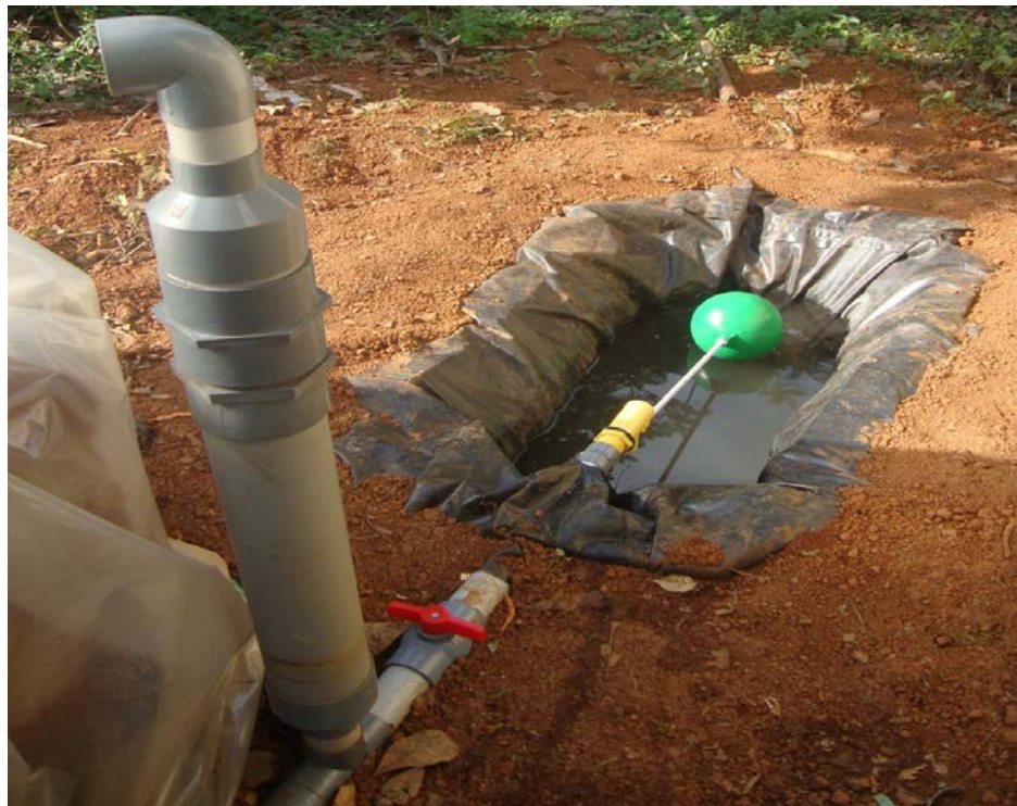
Plate 4.3 First flush diversion system
