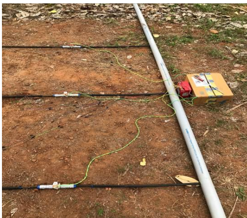
Plate 3.200 Automation Components setup
