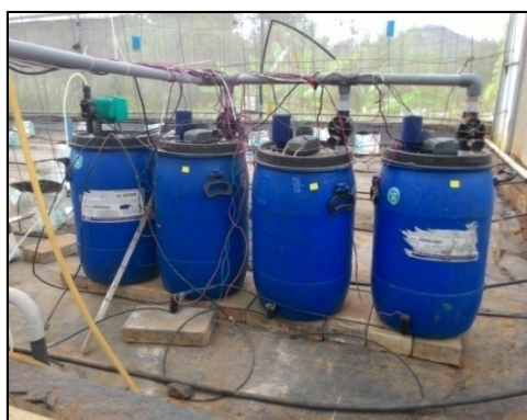
Plate 3.10 Fertilizer tank along with mixing tank and FIP arrangement
