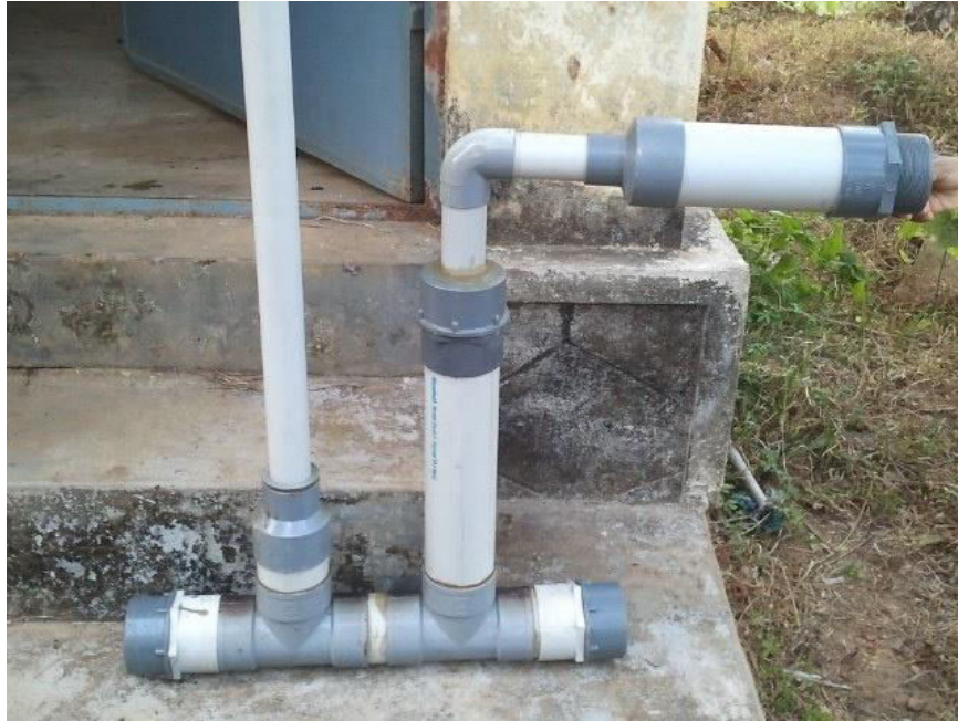
Plate 3.1 Experimental setup of roof water purification
