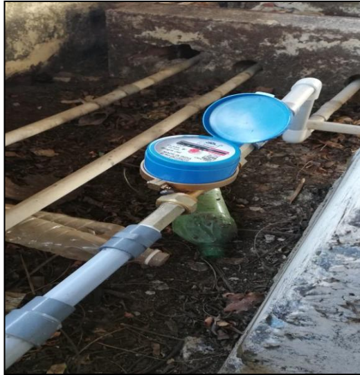
Fig. 3.11 Water Meter at Staff Apartment
