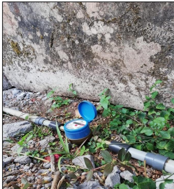
Fig. 3.6 Water meter at Canteen
