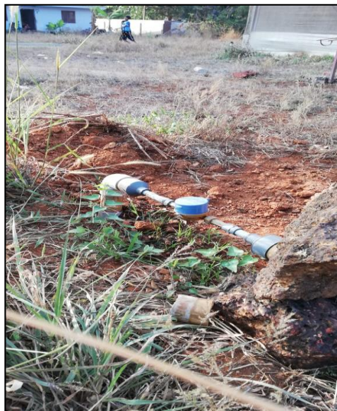
Fig. 3.10 Water Meter at Staff Duplex
