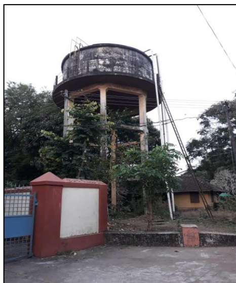
Fig. 3.5 Overhead tank near Ladies' Hostel
