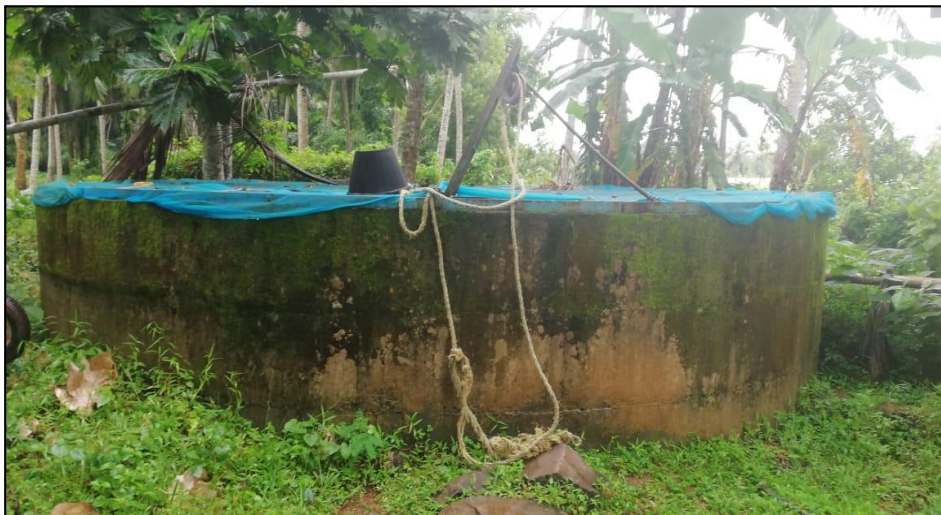
Fig. 3.1 Open well near farm office: 10.854934 N, 75.9858506 E
