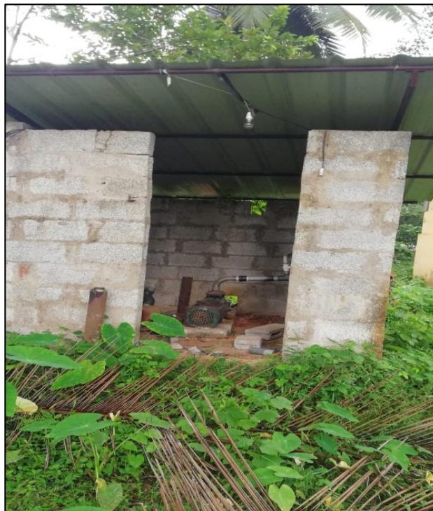
Fig 3.3 Bore well with centrifugal pump: 10.856614 N, 75.884458 E
