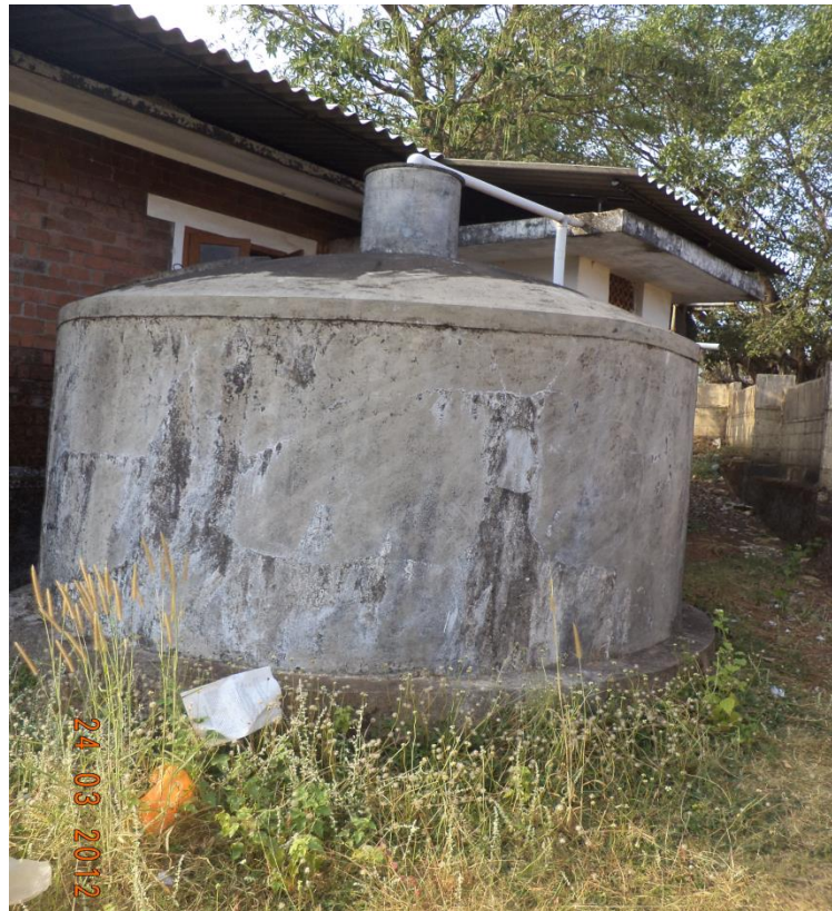
Fig. 4.1 Roof water harvesting system in the village office, Tavanur
