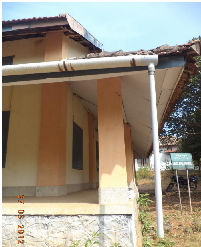
Fig. 4.5 Gutter and conveyance system of RRWHS near library, KCAET, Tavanur
