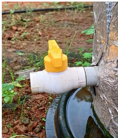
Plate 3.10 Ball valve fitted at the bottom of supply tank
