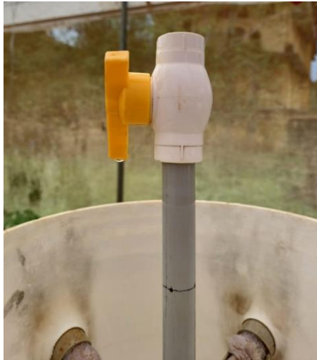
Plate 3.9 Ball valve fitted at the end of vertical PVC
