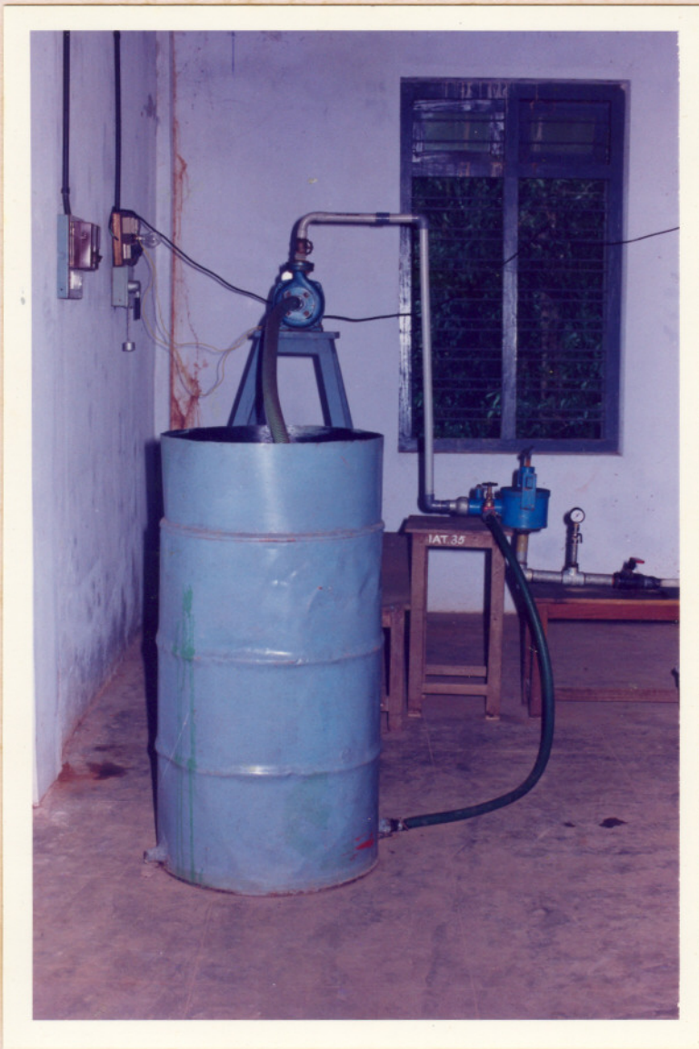
Plate 2 View of the control head
