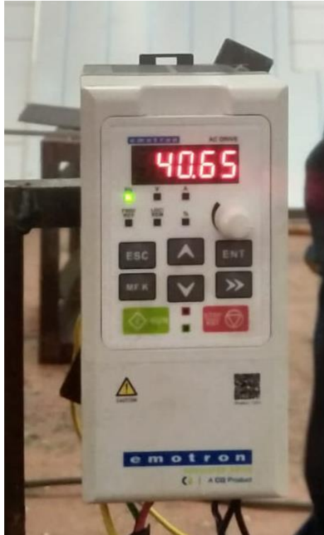
Plate 3.13 Variable Frequency Drive (VFD)
