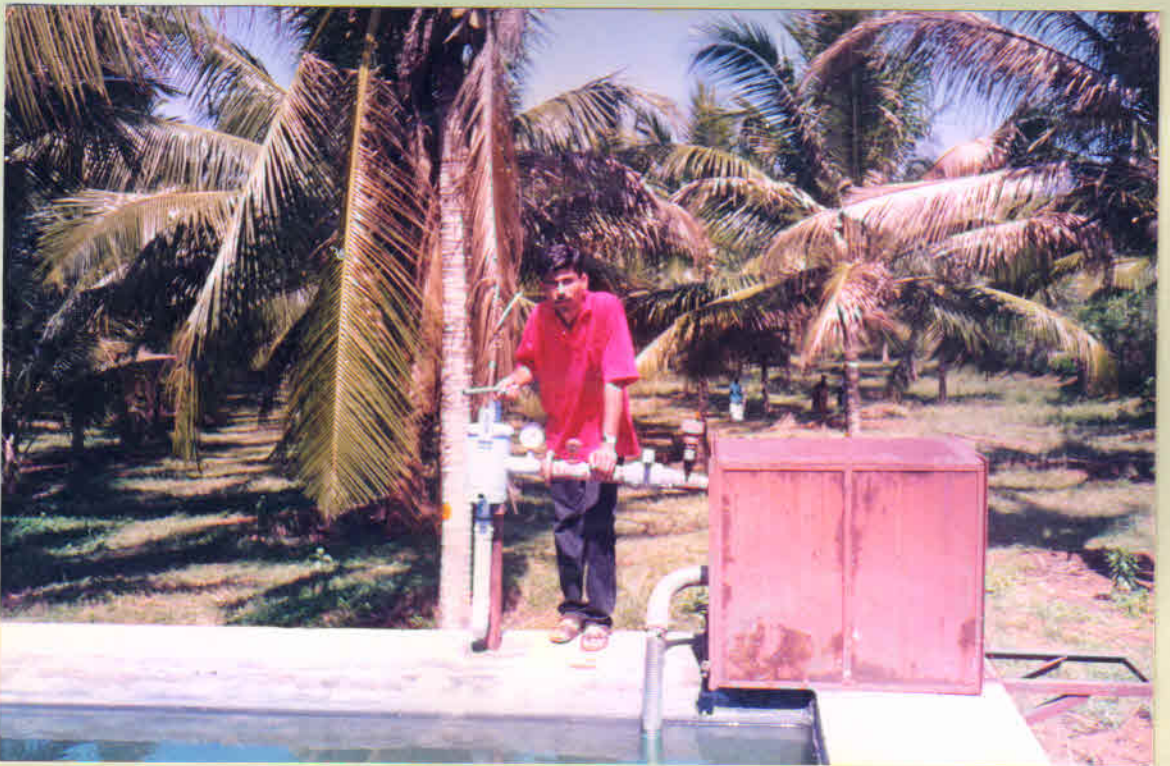
THE HEAD ASSEMBLY OF DRIP IRRIGATION SYSTEM AT WMUTC, VELLANIKKARA
