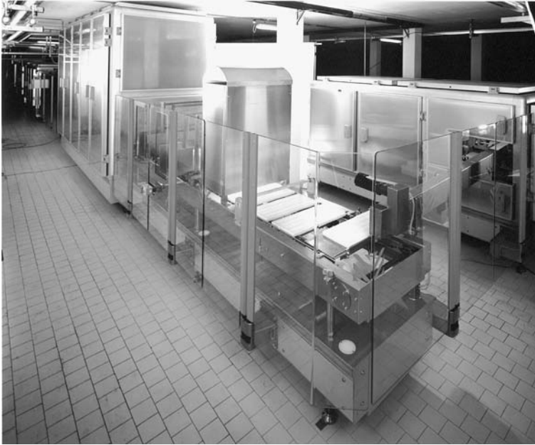
Figure 14.2 Picture of turning point on loose mould moulding plant (OPM Italy).
