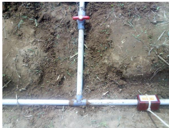
Plate 4. Magnetic fluid conditioner attached to control line
