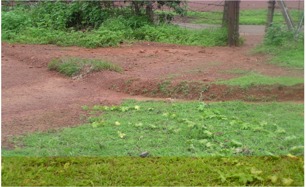
Plate. 2 Interceptor drain at the eastern side
