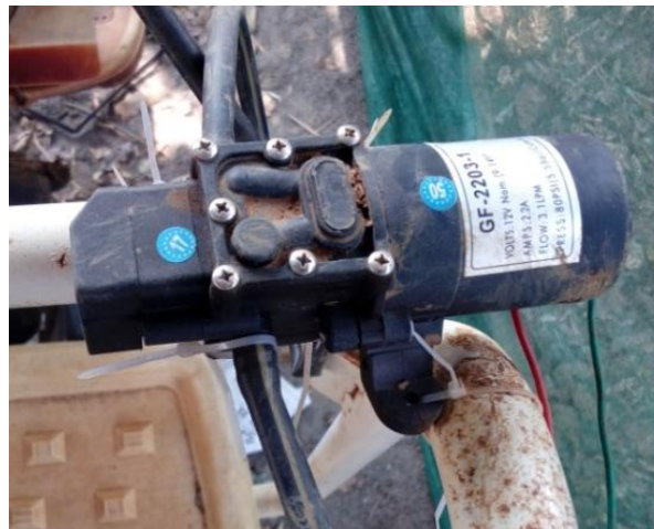
Figure 4.9 Battery operated 12 V pump
