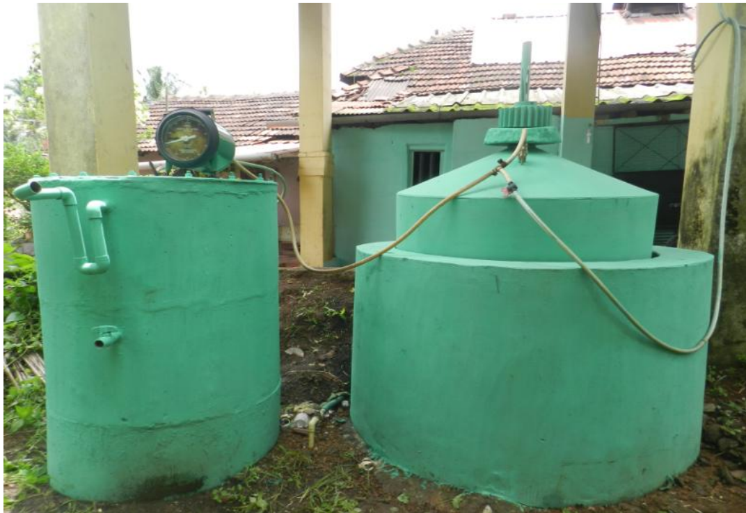
Plate 3.6 Full scale UAHBR installed at Edible Oil Mill, Pattambi
