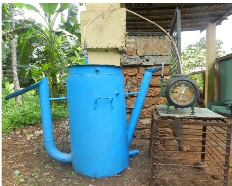
Plate 3.5 Floating gas holder digester with wet gas flow meter installed at oil mill
