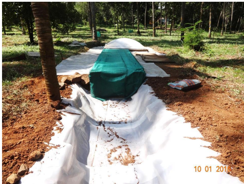
Plate 4.1 Filter unit with conveying channel
