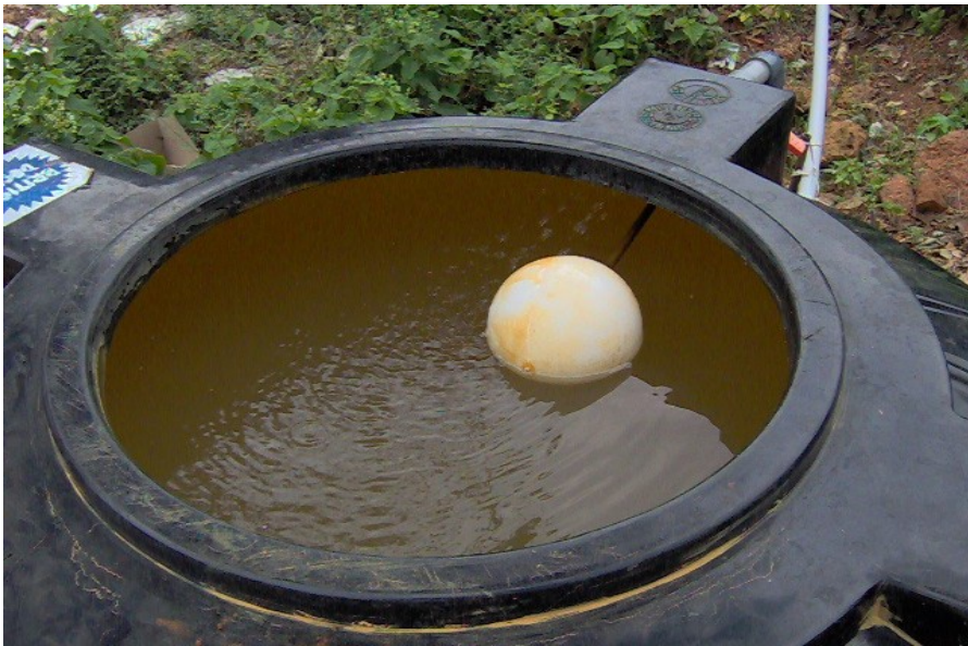
Plate 3.7. Feeder Tank with Float Valve
