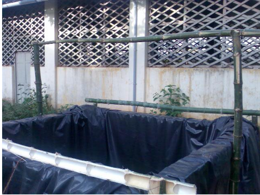
Figure 4.5 Storage tank, lined with HDPE sheet
