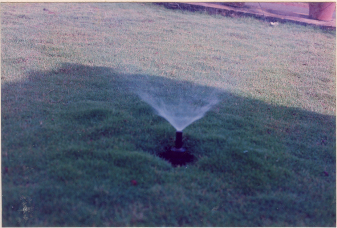
PLATE 3 - POP-UP SPRINKLER IN OPERATION
