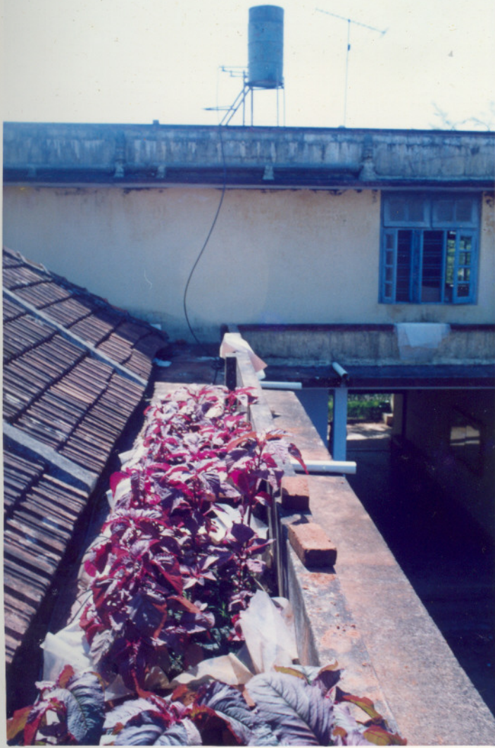
Plate 1. View of the storage tank for drip irrigation
