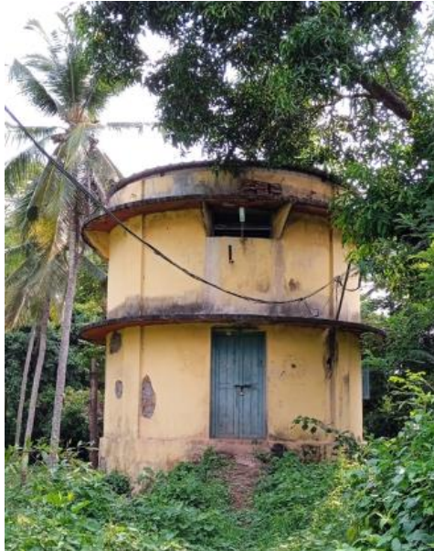
Plate4.1 Intake well with pumphouse
